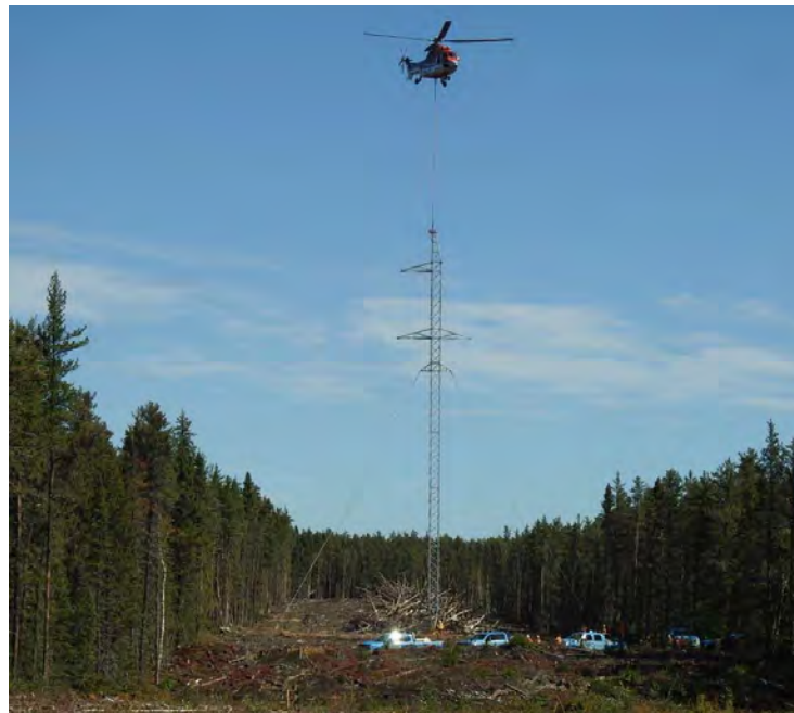
Helicopter holding the tower in place while the ground crew connects guy wires.
