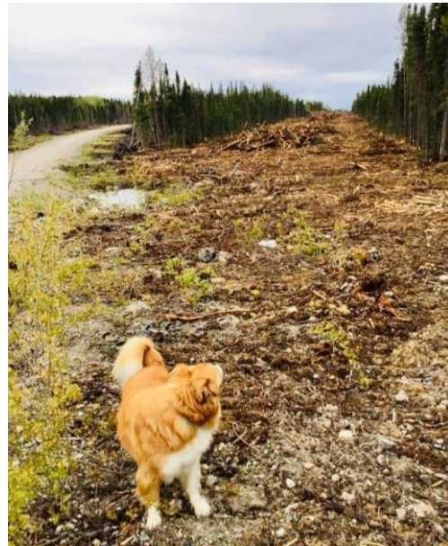
"Mr. Man" checking out the cleared right of way. (Photo credit: David Jeremiah, Community Liaison)
